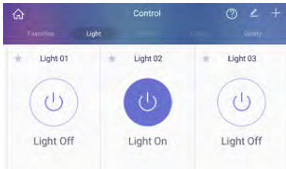
[Lighting Control Screen]
